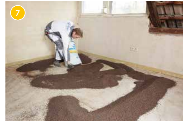
Raise two parallel banks at the desired levelling height, lay levelling boards on them and align the latter.
