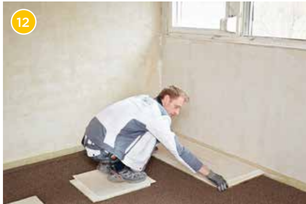
Now start laying the Rigidur flooring elements in the back left corner of the room. If necessary, lay out stepping surfaces made of Rigidur flooring elements to avoid stepping on the dry compound.
