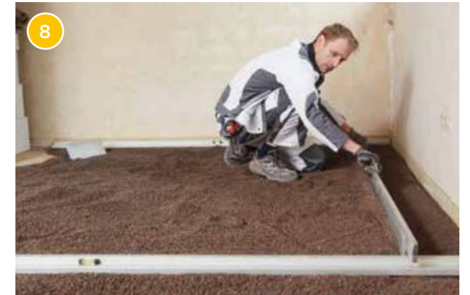
Smooth out and level the surface with a smoothing gauge over the levelling boards. Then remove the boards.
