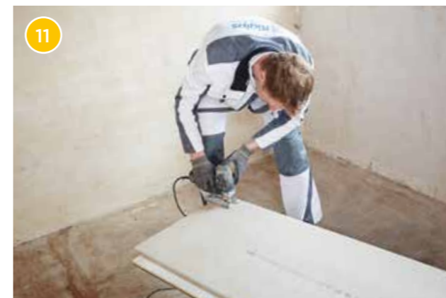
Cut the rebate edges off the first flooring element at the wall connections of the longitudinal and transverse side.
