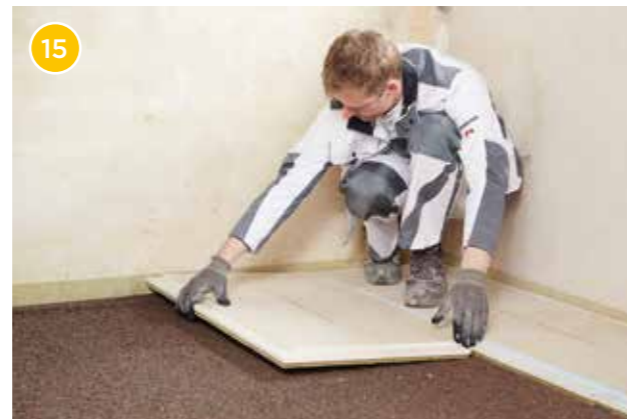
Now lay more Rigidur flooring elements and screw the elements in rows throughout. The transverse joints of the elements must be at least 20 cm apart.
