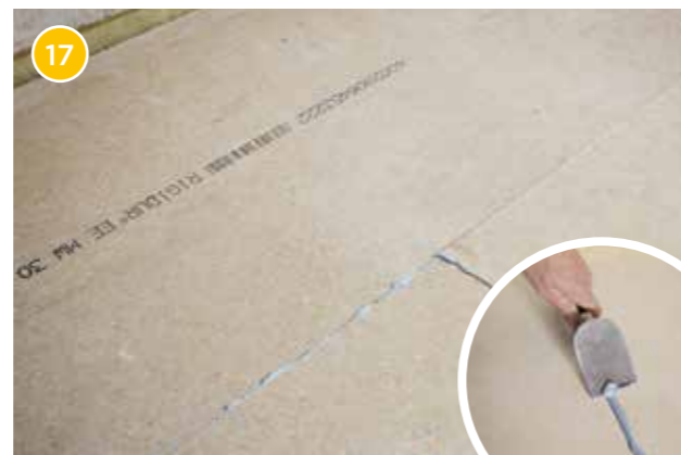
Residual adhesive can be scraped off along the joint to create a smooth and flat surface. The adhesive will have hardened fully after approx. 24 hours and floor coverings can be laid.
